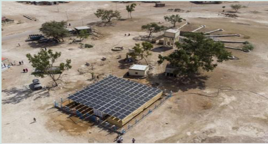
Figure 3: The 6 m 3 /h solar powered reverse osmosis water desalination facility implemented by Genius Watter Srl in Ainabo, Somalia (Rossi, 2023).
